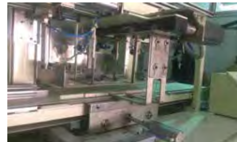
V Engineering, Surendra Shelke, Pune, India Verpackungsmaschine Packing machine
