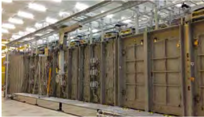
Applied Materials, Chung cheng Chen, Tainan City, Taiwan Testmaschine Testing machine
