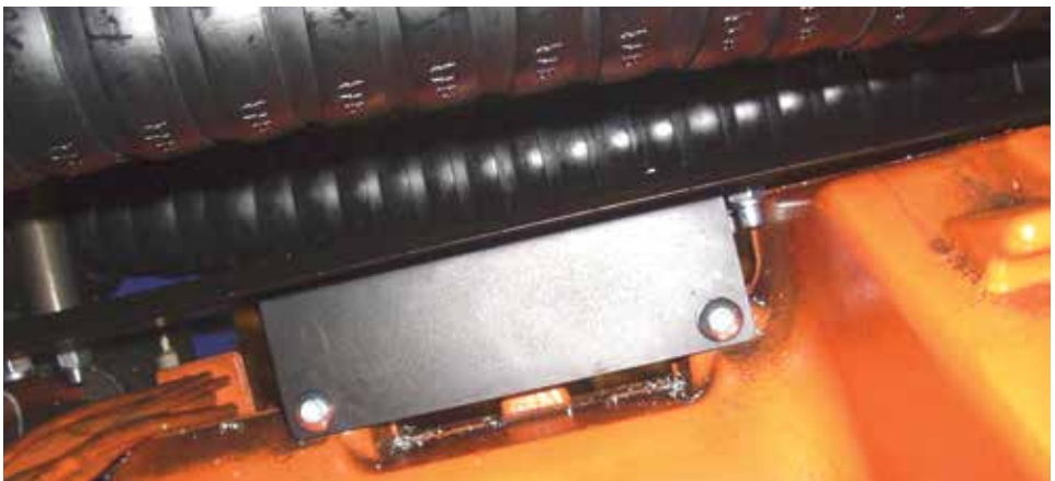
Application example with RS system on ABB Series 6600
